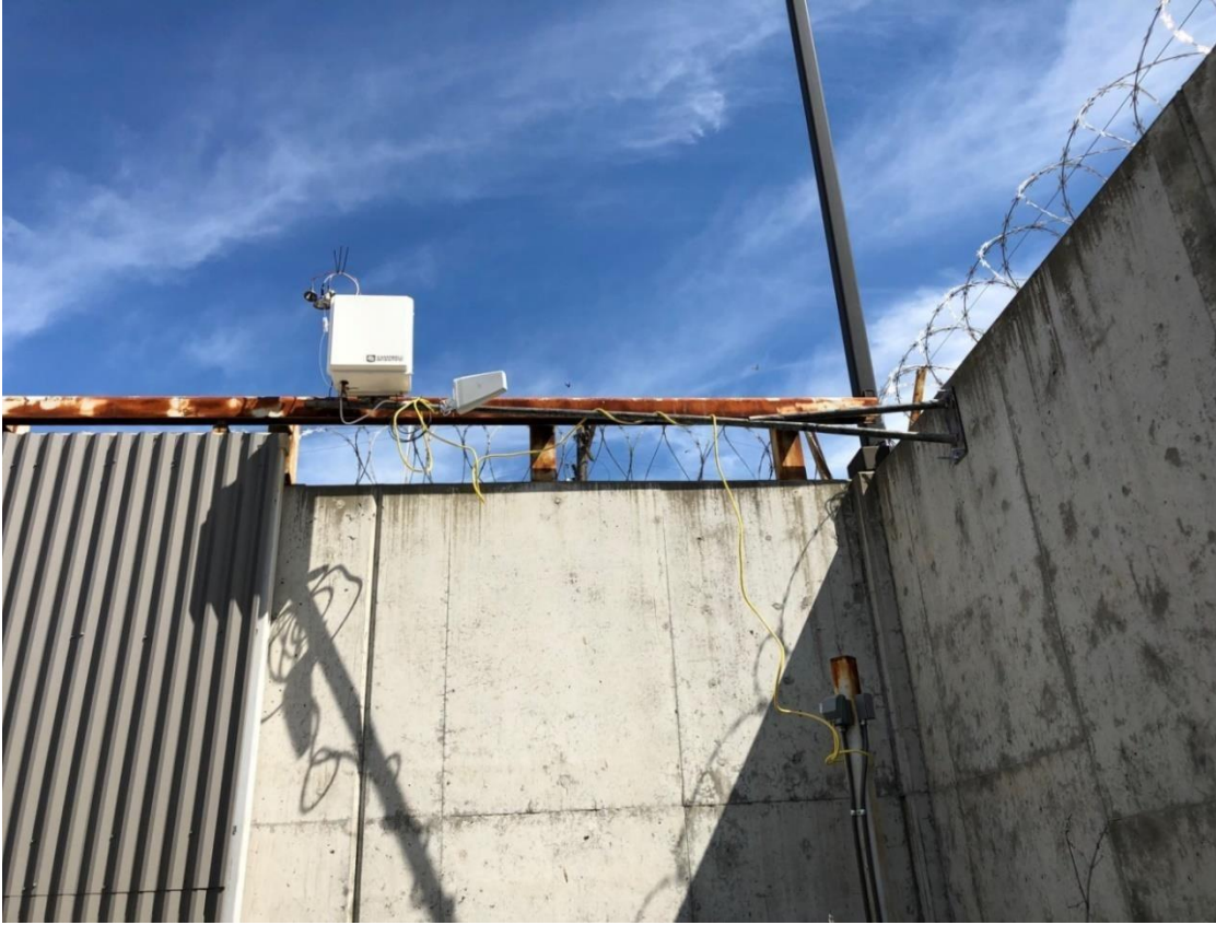
Figure 4. Site 3 Monitoring System
